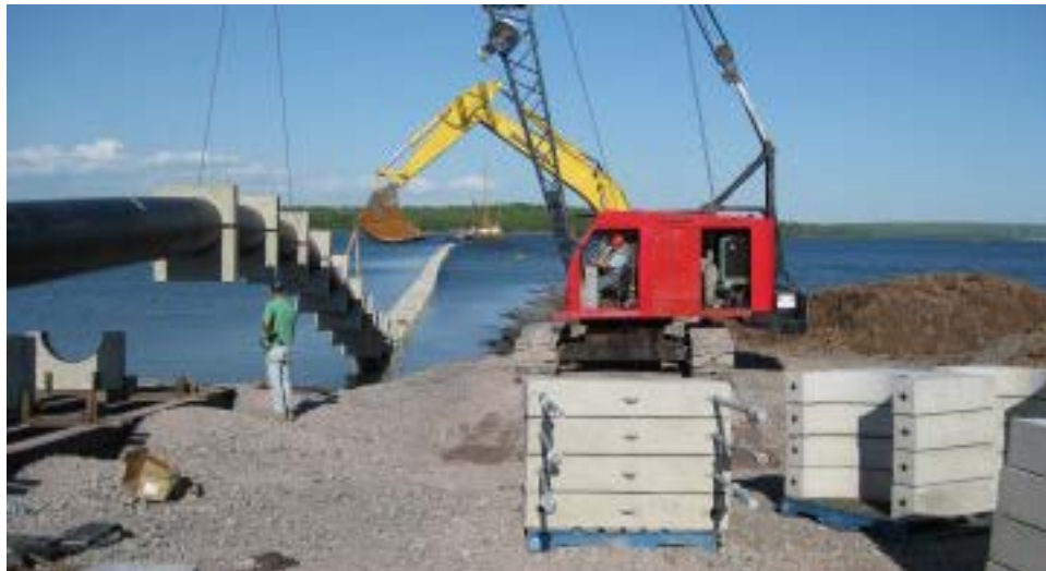
Figure 26. Image of pipeline being pulled into Pictou Harbor, 2009, images courtesy of Northern Pulp.
