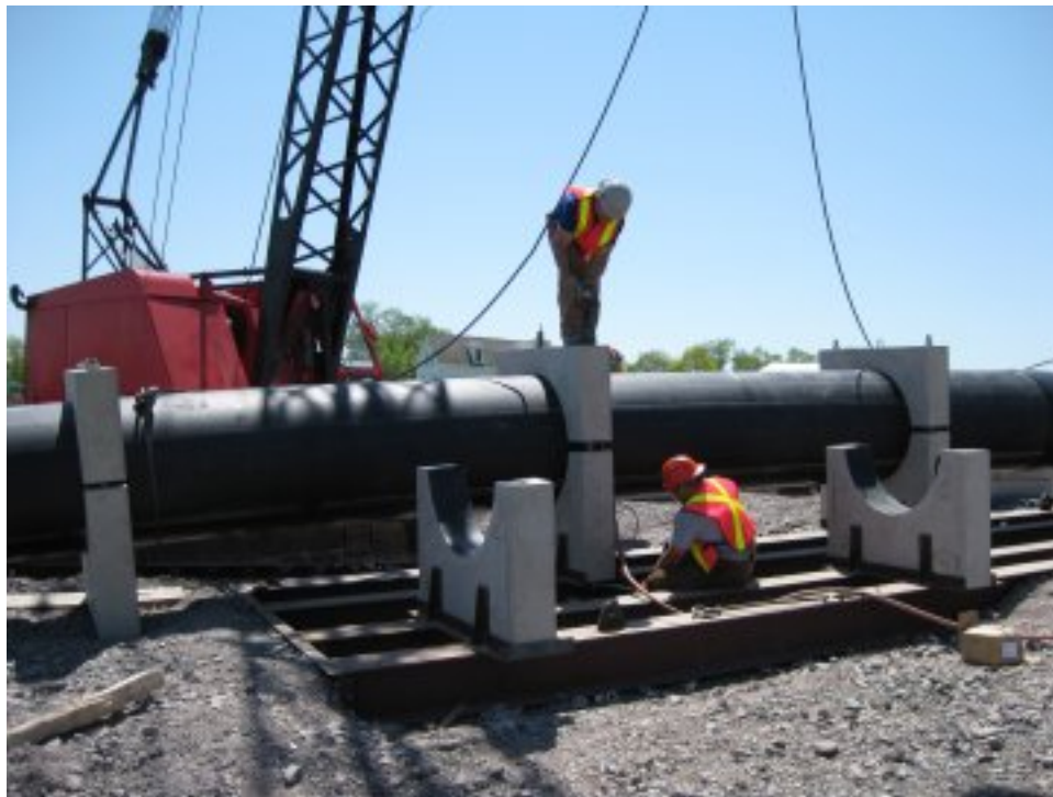
Figure 27. Image of pipe weights being affixed to HDPE pipeline prior to deployment at Pictou Harbor, 2009, images courtesy of Northern Pulp.
