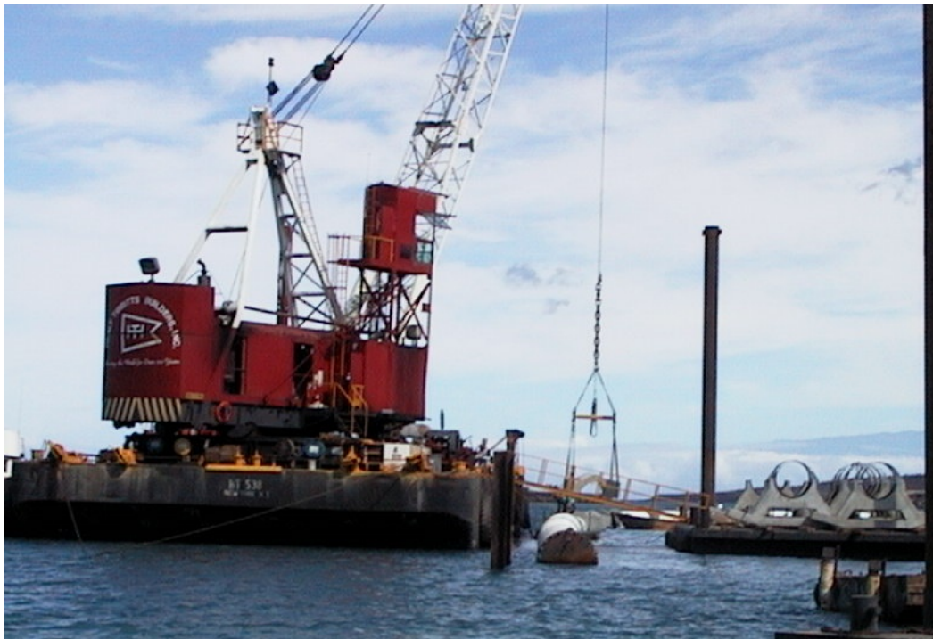
Figure 32. Pipe weights being installed on floating pipeline using a crane barge with an elevator mounted on its side.
