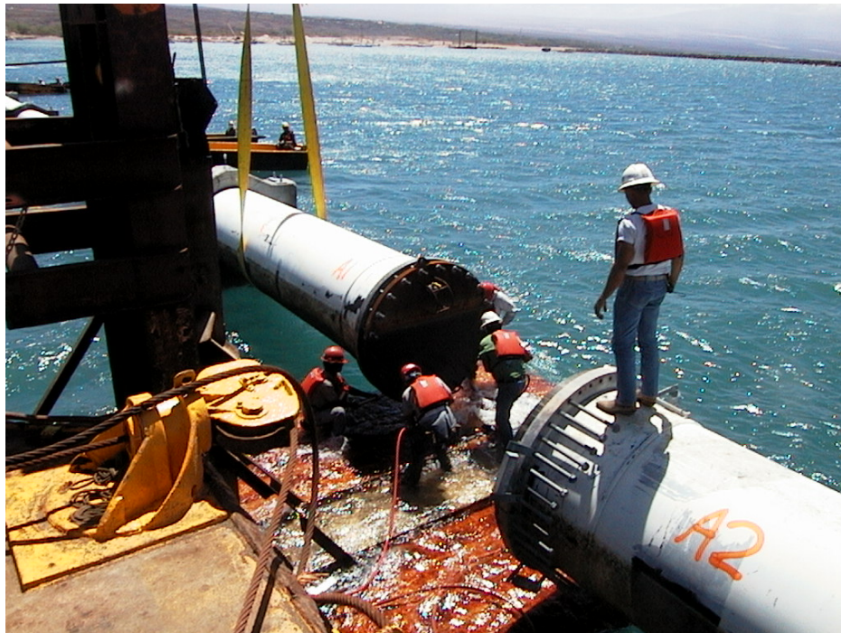
Figure 33. View of elevator platform mounted on a barge – here used for flange connections on 55” pipe in Hawaii 2001.
