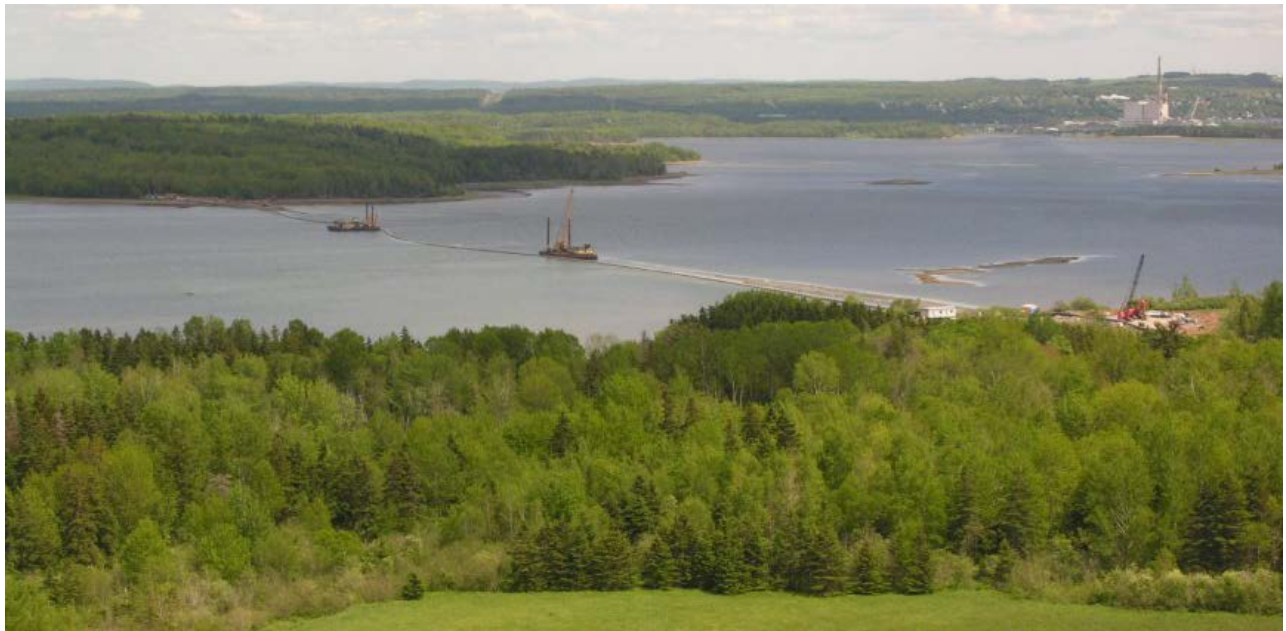
Figure 8. Staged pipeline towed into Pictou Harbor from Northern Pulp Mill, 2009, images courtesy of Northern Pulp.
