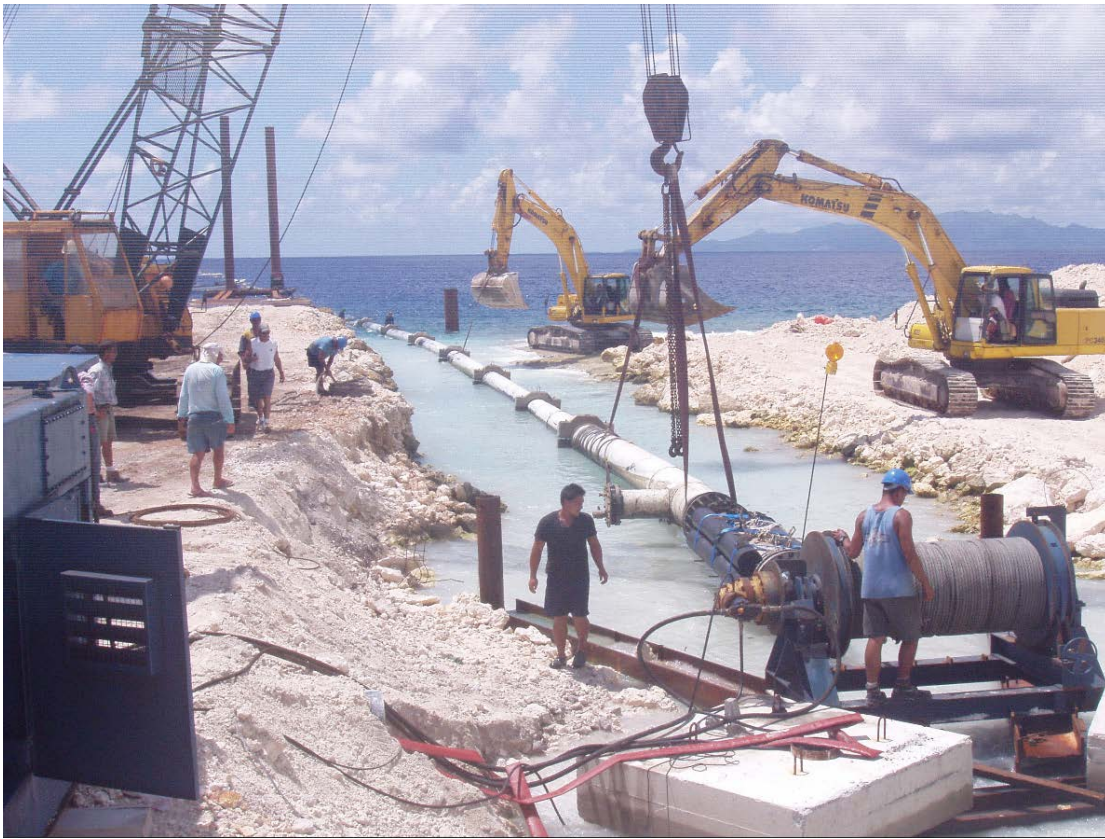
Figure 34. Completed pipe trench with pipe pulled in from offshore by shore winch.
